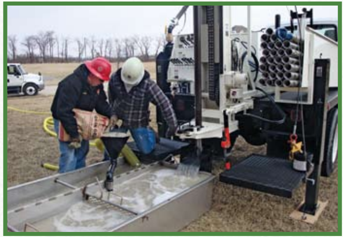
The only rule of thumb in geothermal installation is that no two jobs are alike. You will need a toolbox full of solutions to solve each project, including mud mixers, grouts and drilling fluids.
